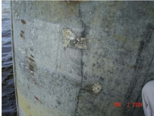
Figure 3.4 Longitudinal crack in prestressed concrete cylinder pile.
