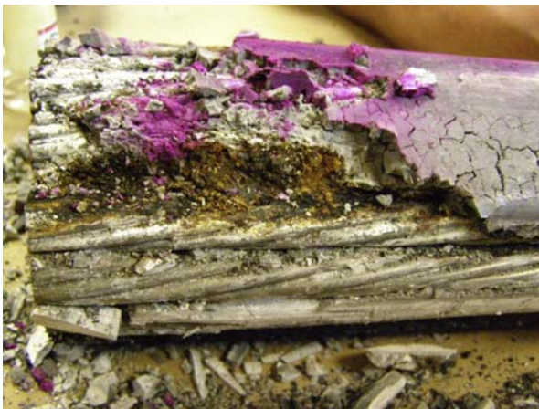
Figure 3.5 Corrosion of a strand embedded in deficient grout. Pink color shows the pH indicator (phenolphthalein) sprayed on the grout surface.
