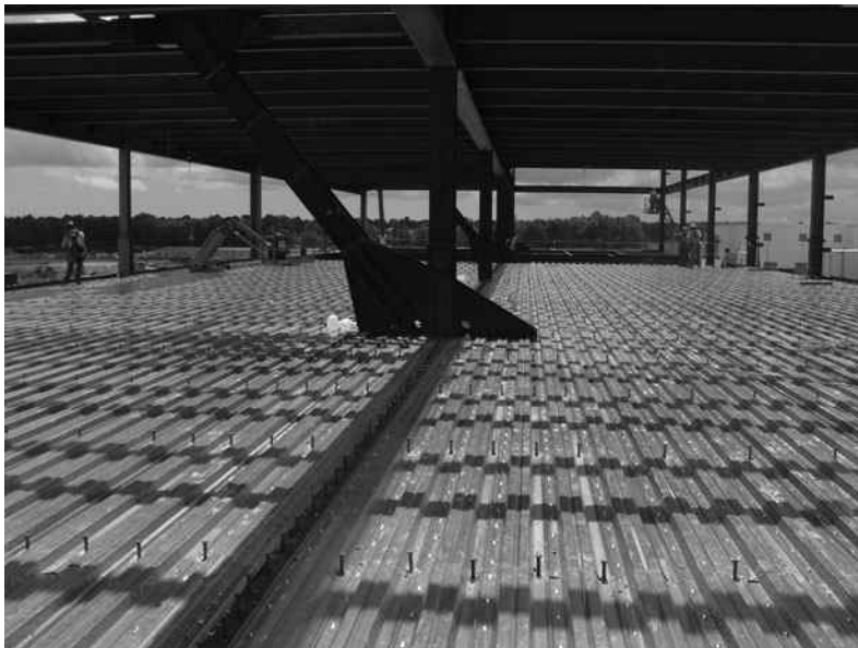
Composite floor framing, North Charleston, SC. (Courtesy of CMC South Carolina Steel.)
