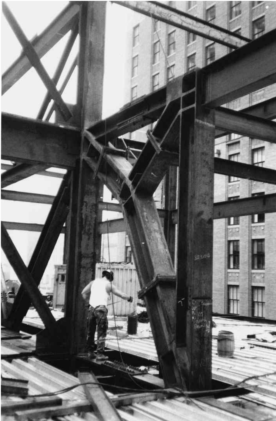
Transfer truss, 150 Federal Street, Boston, MA. (Courtesy of Owen Steel Company, Inc.)
