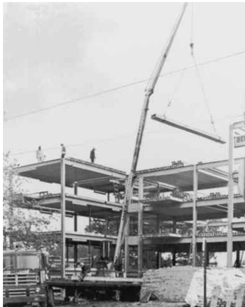
Interns' living quarters, Good Samaritan Hospital, Dayton, OH. (Courtesy of Flexicore Company, Inc.)
