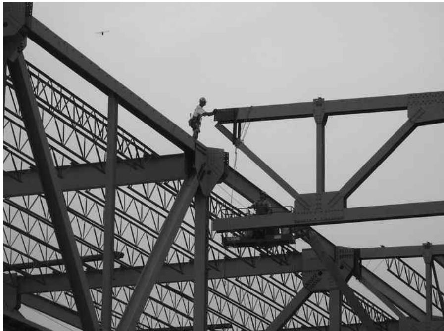
Erection of roof truss, North Charleston, SC. (Courtesy of CMC South Carolina Steel.)
