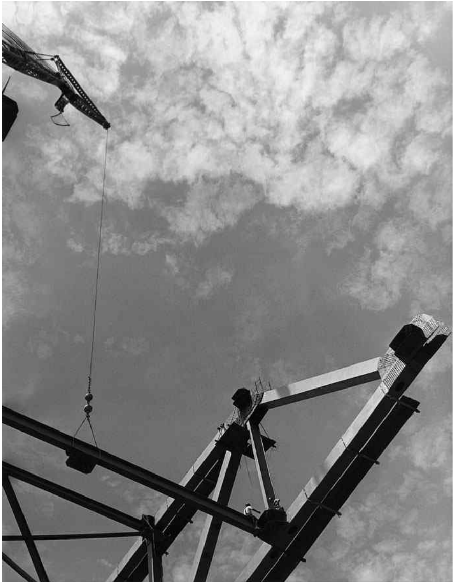
Bridge over Allegheny River at Kittanning, PA. (Courtesy of the American Bridge Company.)
