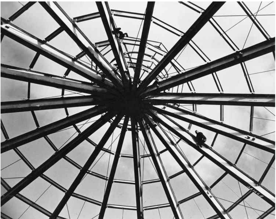
The skeleton of the roof of a Ford building under construction. (Courtesy of Bethlehem Steel Corporation.)
