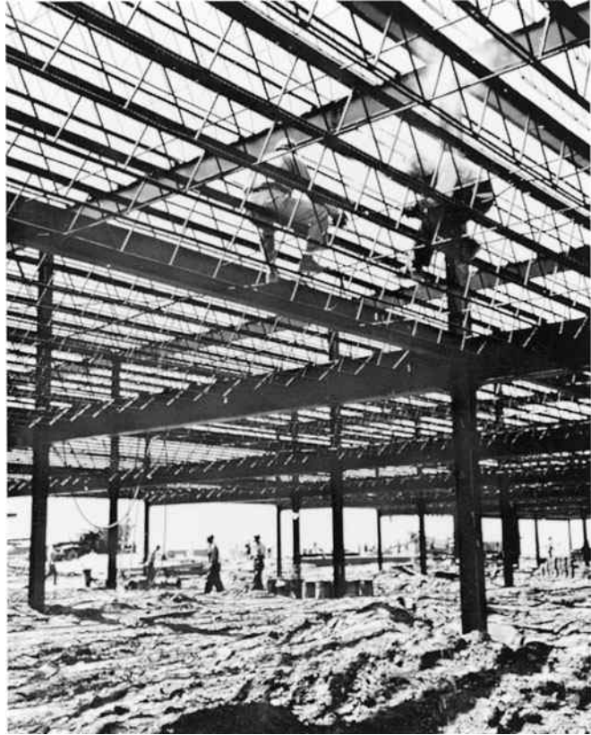
Short-span joists in the Univac Center of Sperry-Rand Corporation, Blue Bell, PA. (Courtesy of Bethlehem Steel Corporation.)
