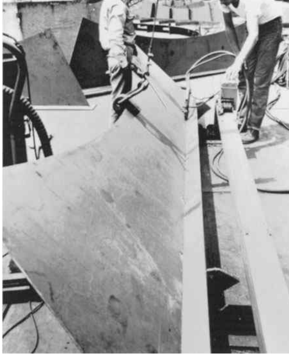
Lincoln ML-3 Squirtwelder mounted on a self-propelled trackless trailer deposits this 1/4-in web-to-flange weld at 28 in/min. (Courtesy of the Lincoln Electric Company.)
