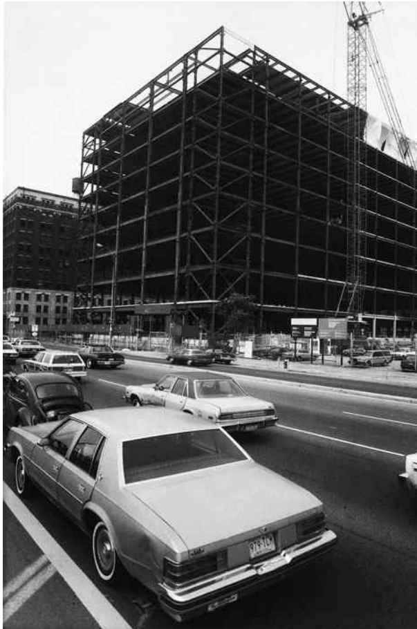
Shearson Lehman/American Express Information Services Center, New York City. (Courtesy of Owen Steel Company, Inc.)
