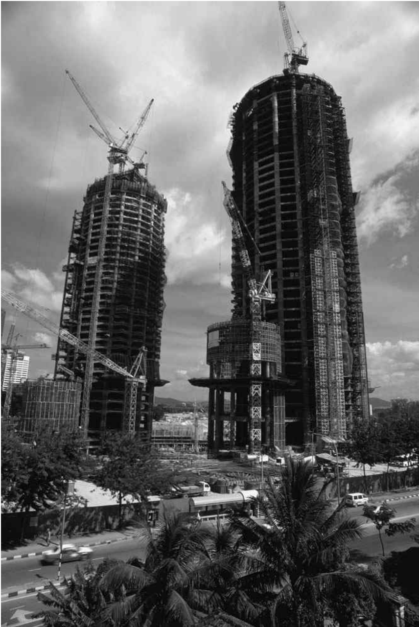
Construction of the twin Petronas Towers in Kuala Lumpur, Malaysia. (Courtesy of Corbis/Sergio Dolzntes.)
