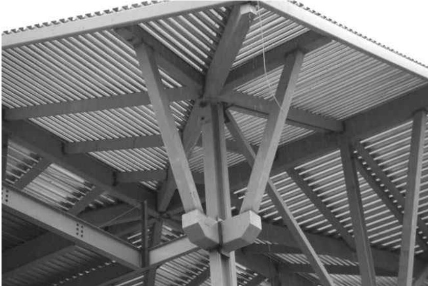
Roof framing for Cherokee Central Schools, Cherokee, NC. (Courtesy of CMC South Carolina Steel.)
