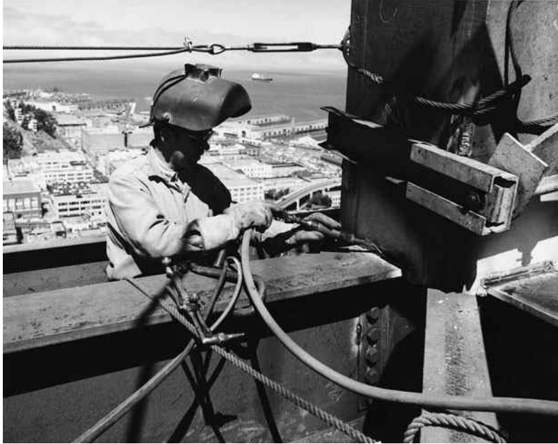
Combined welded and bolted joint, Transamerica Pyramid, San Francisco, CA. (Courtesy of Kaiser Steel Corporation.)
