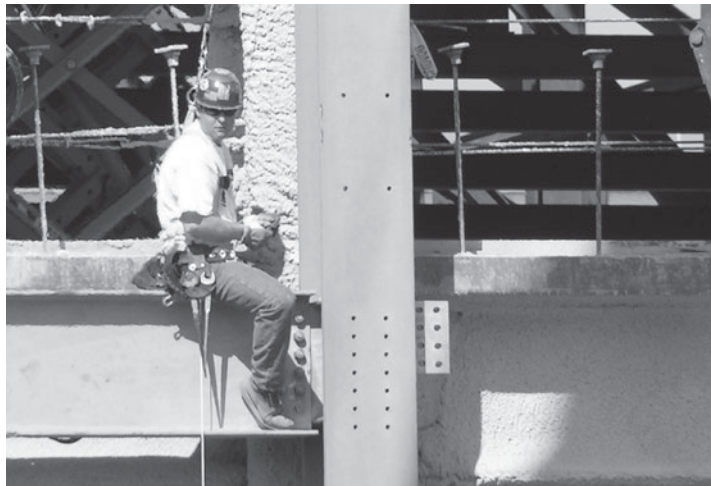
An ironworker awaits the lifting of a steel beam that will be field bolted to the column. (Courtesy of CMC South Carolina Steel.)
