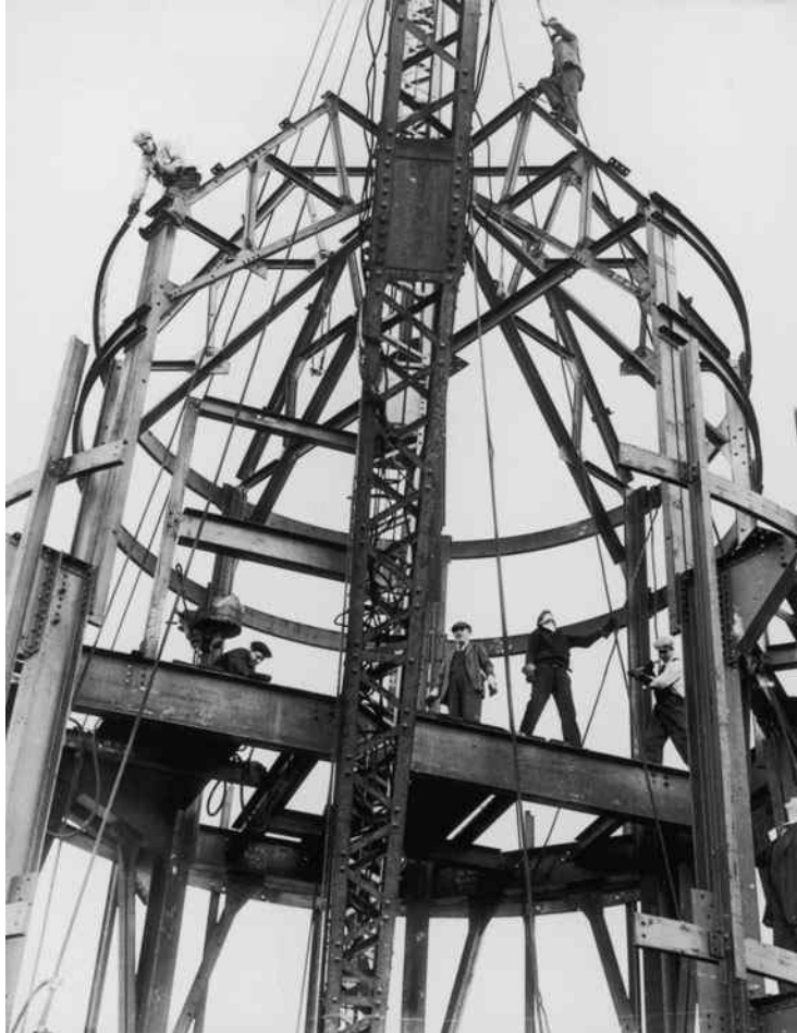
The mooring mast of the Empire State Building, New York City. (Courtesy of Getty Images/Hulton Archive Photos.)
