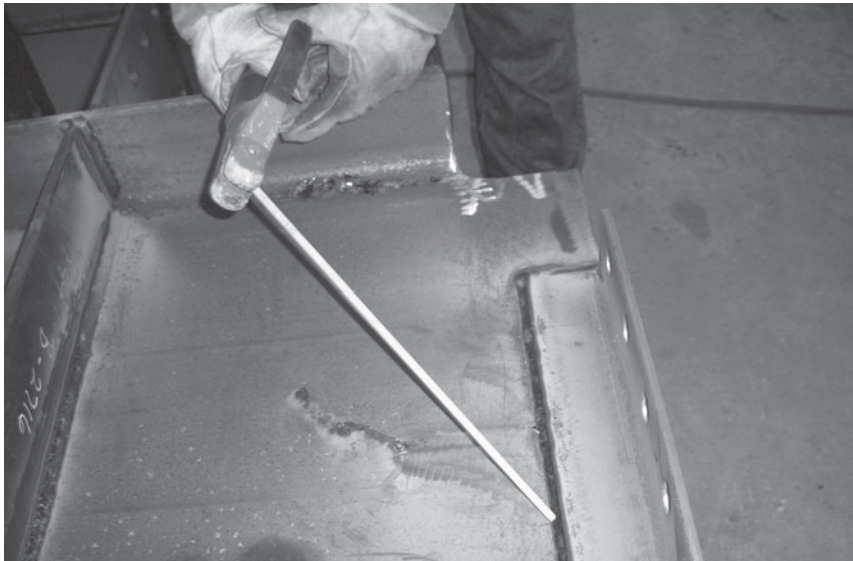
Shielded metal arc welding (SMAW) and electrode just before starting an arc to fillet weld the clip angle to the beam web. (Courtesy of CMC South Carolina Steel.)
