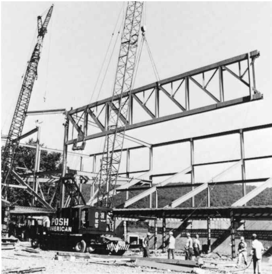
One-half of a 170-ft clear span roof truss for the Athletic and Convention Center, Lehigh University, Bethlehem, PA. (Courtesy of Bethlehem Steel Corporation.)
