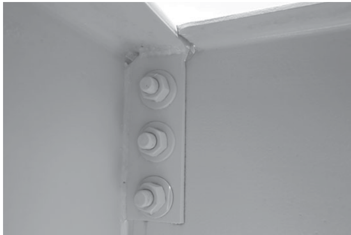
A shear tab, or single-plate, framing connection. (Picture taken by the author.)
