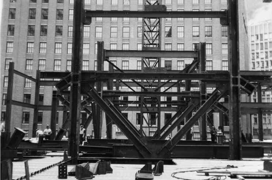
Transfer truss, 150 Federal Street, Boston, MA. (Courtesy Owen Steel Company, Inc.)
