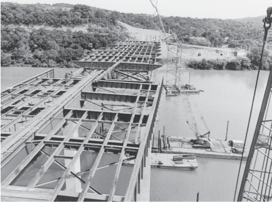
Bridge over Allegheny River at Kittanning, PA. (Courtesy of the American Bridge Company.)
