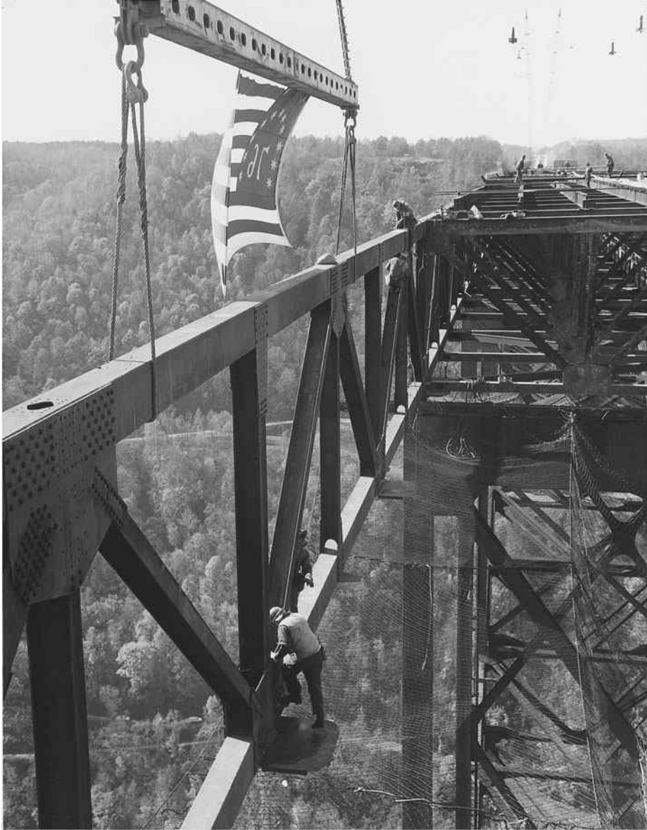
Bridge over New River Gorge near Charleston in Fayette County, WV. (Courtesy of the American Bridge Company.)
