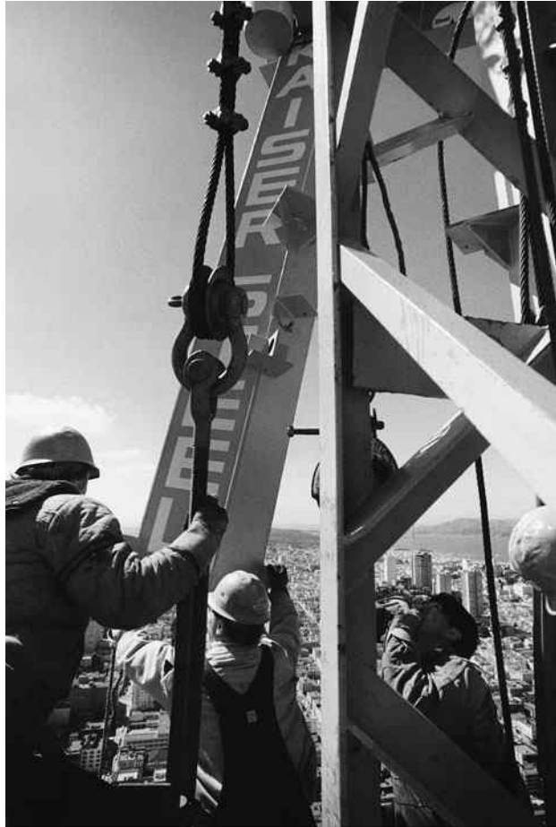
Steel erection for Transamerica Pyramid, San Francisco, CA. (Courtesy of Kaiser Steel Corporation.)
