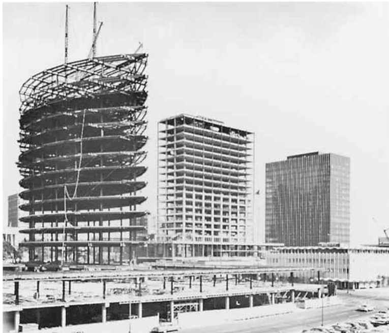
Three high-strength bolted structures in Constitution Plaza Complex, Hartford, CT, using approximately 195,000 bolts. (Courtesy of Bethlehem Steel Corporation.)
