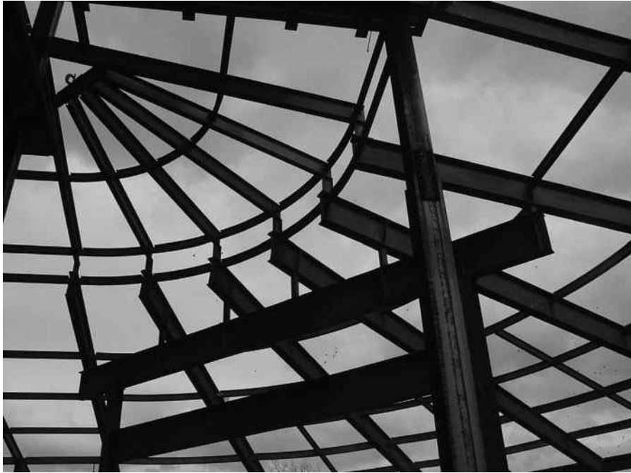
Roof framing for Glen Oaks School, Bellerose, NY. (Courtesy of CMC South Carolina Steel.)
