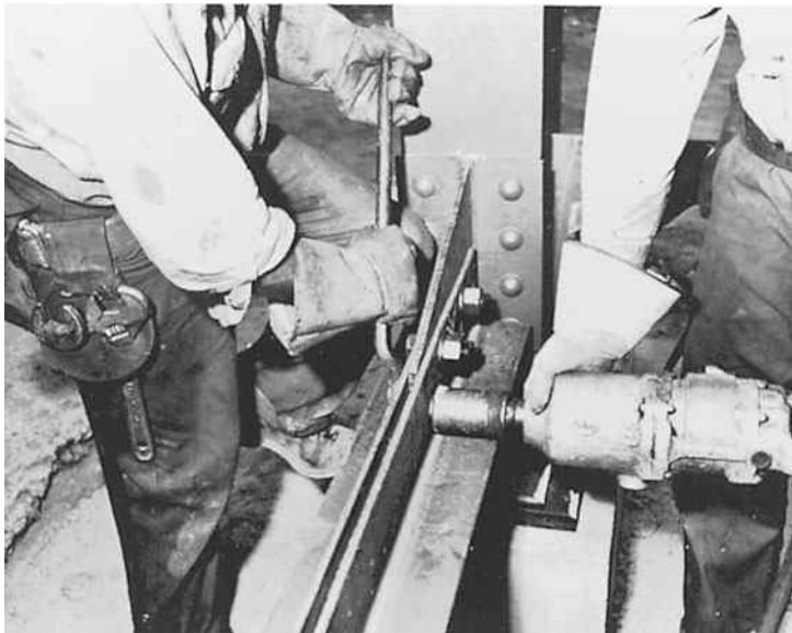
Torquing the nut for a high-strength bolt with an air-driven impact wrench. (Courtesy of Bethlehem Steel Corporation.)
