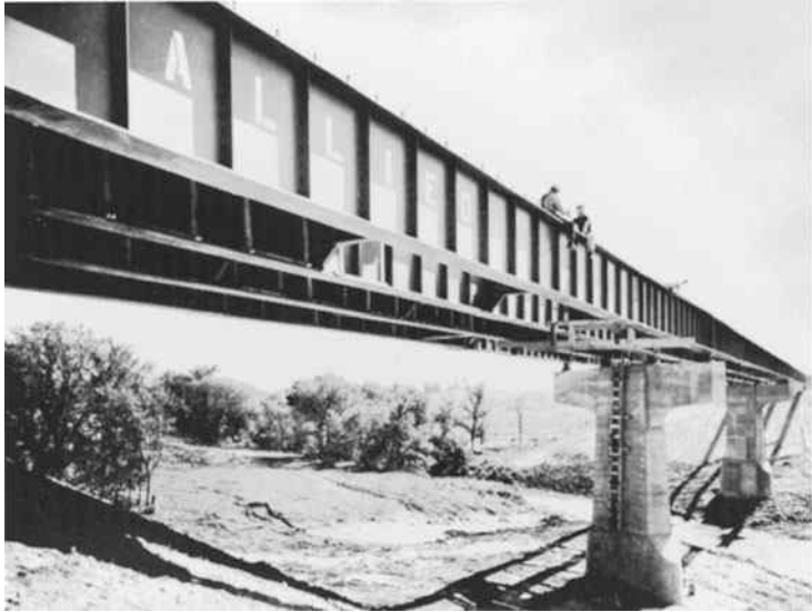
Continuous-welded plate girders in Henry Jefferson County, IA. (Courtesy of the Lincoln Electric Company.)
